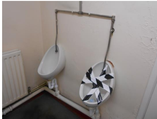
Isolating urinals & wash basins
